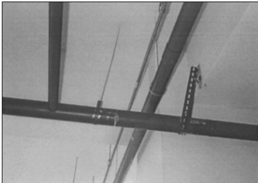
Figure 19 Damage to sprinkler system during the Jiji earthquake in Taiwan
