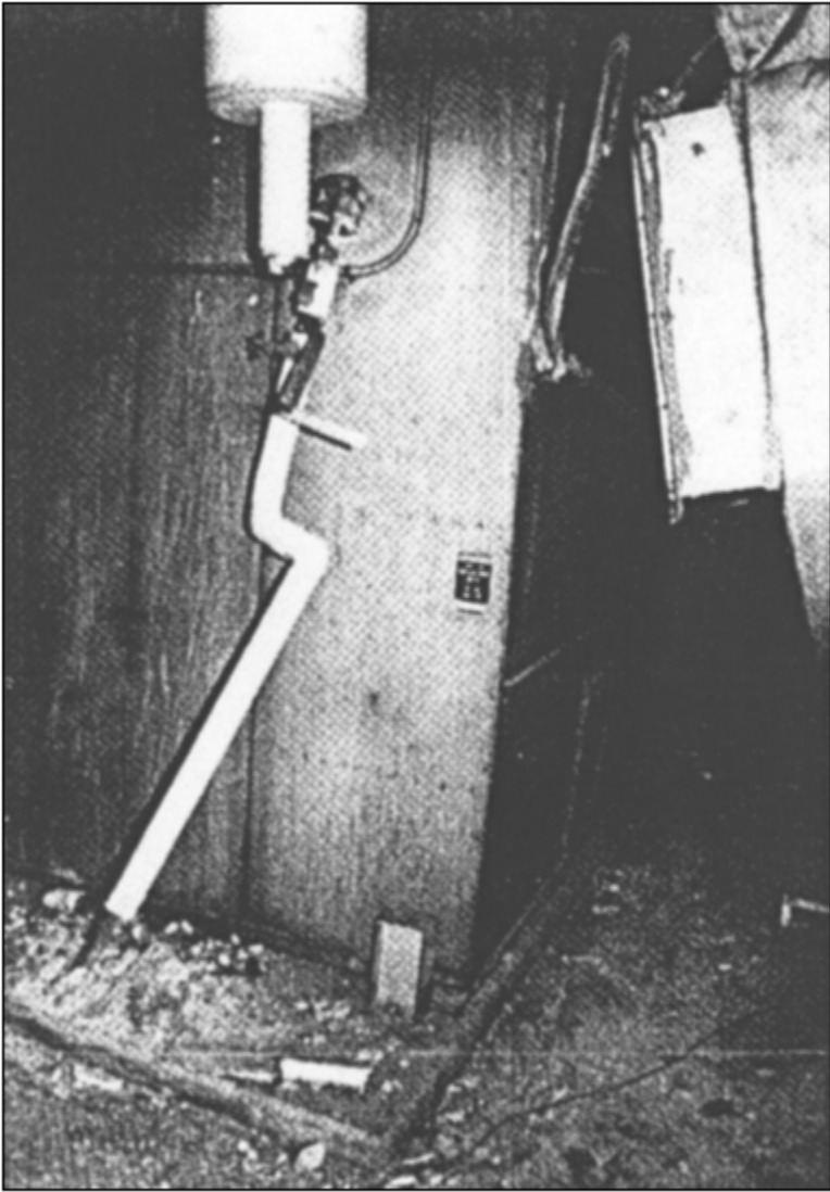
Figure 8 Failure of ducting at ventilation unit during the 1994 Northridge, California earthquake (McKevitt et al., 1995)
