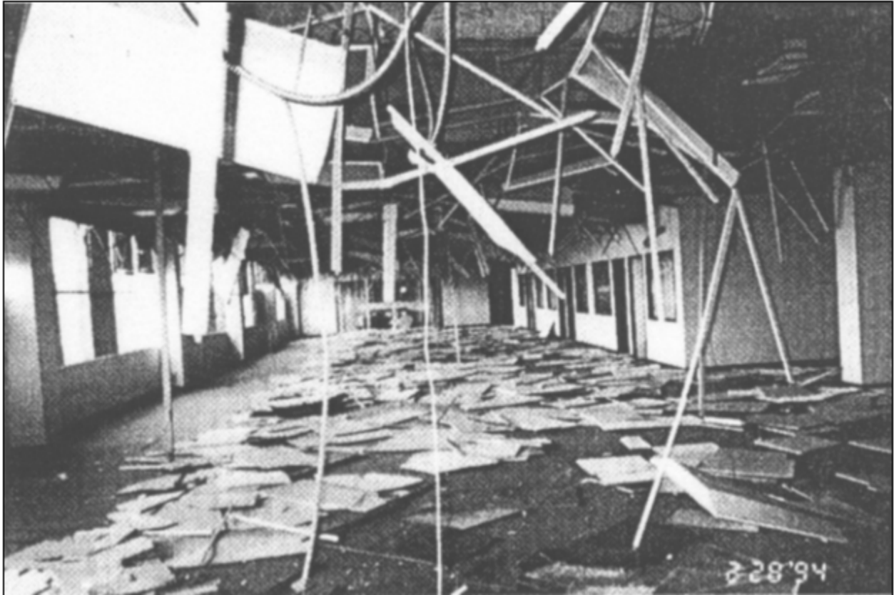
Figure 5 Failure of suspended ceiling and light fixtures during the 1994 Northridge, California earthquake (FEMA 74, 1994)
