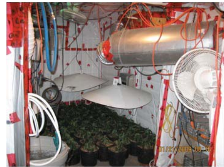
Typical electrical concerns associated with grow operations.
