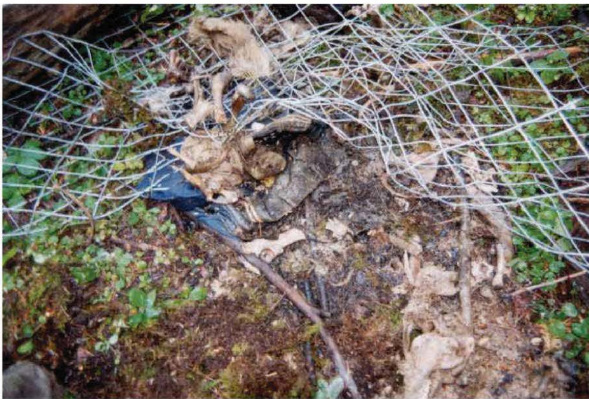
Figure 57 Large Scavenger Damage
